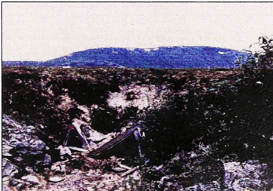
Photograph of lower or western end of the Santa Clara tunnel. Note that timbers are broken and that the near end of tunnel is completely collapsed.
